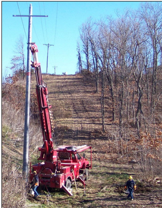
STANDING STRONG...Concrete poles are installed by a West Central Electric contractor along Highway DD between Warrensburg and Knob Noster.
